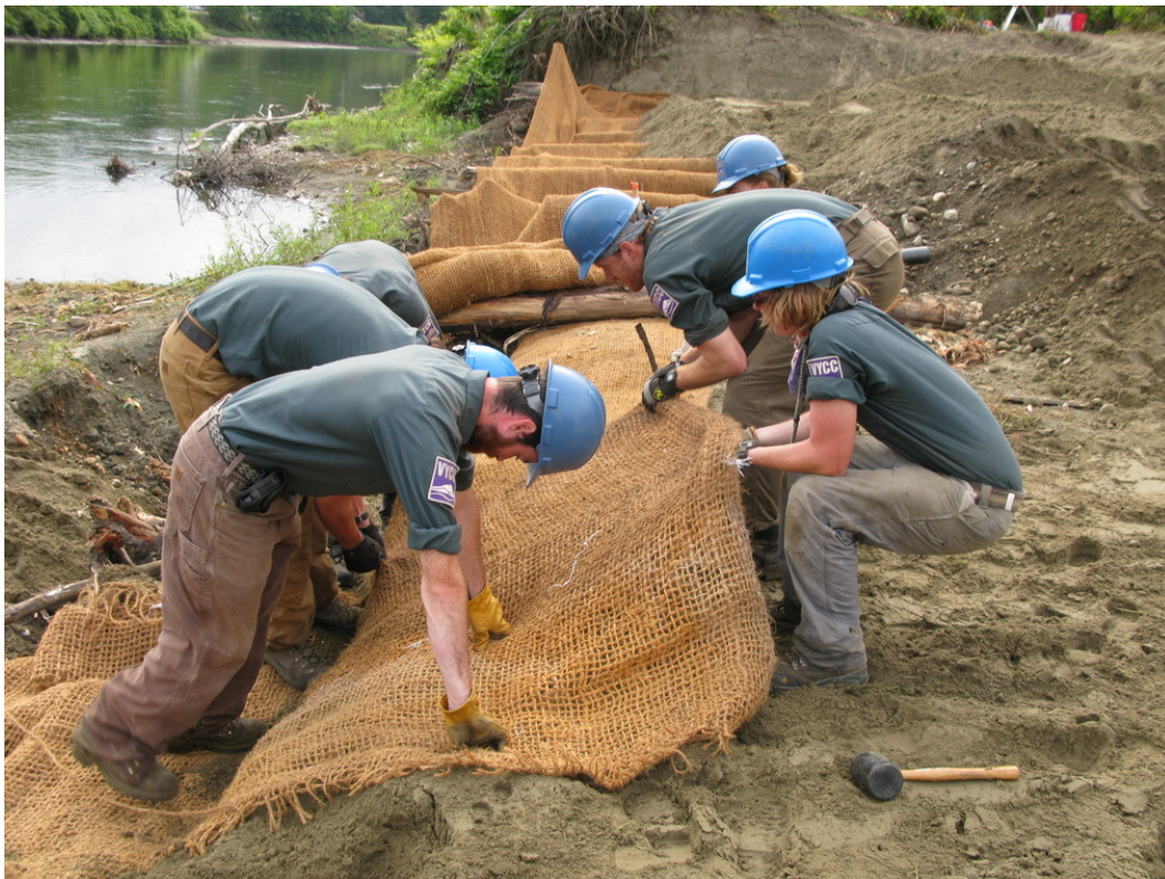
Wrapping coir fabric over compacted soil to create the second soil lift.
