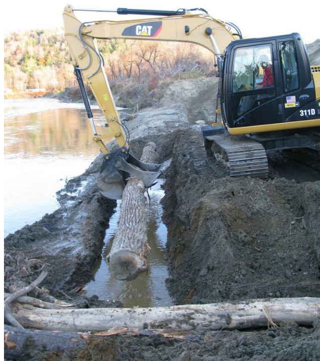
Placing a scour log parallel to and 5-feet back from the river's edge.
