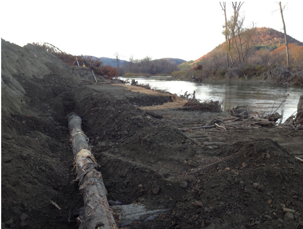
Deadman logs anchor the back of the root wads into the bank.
