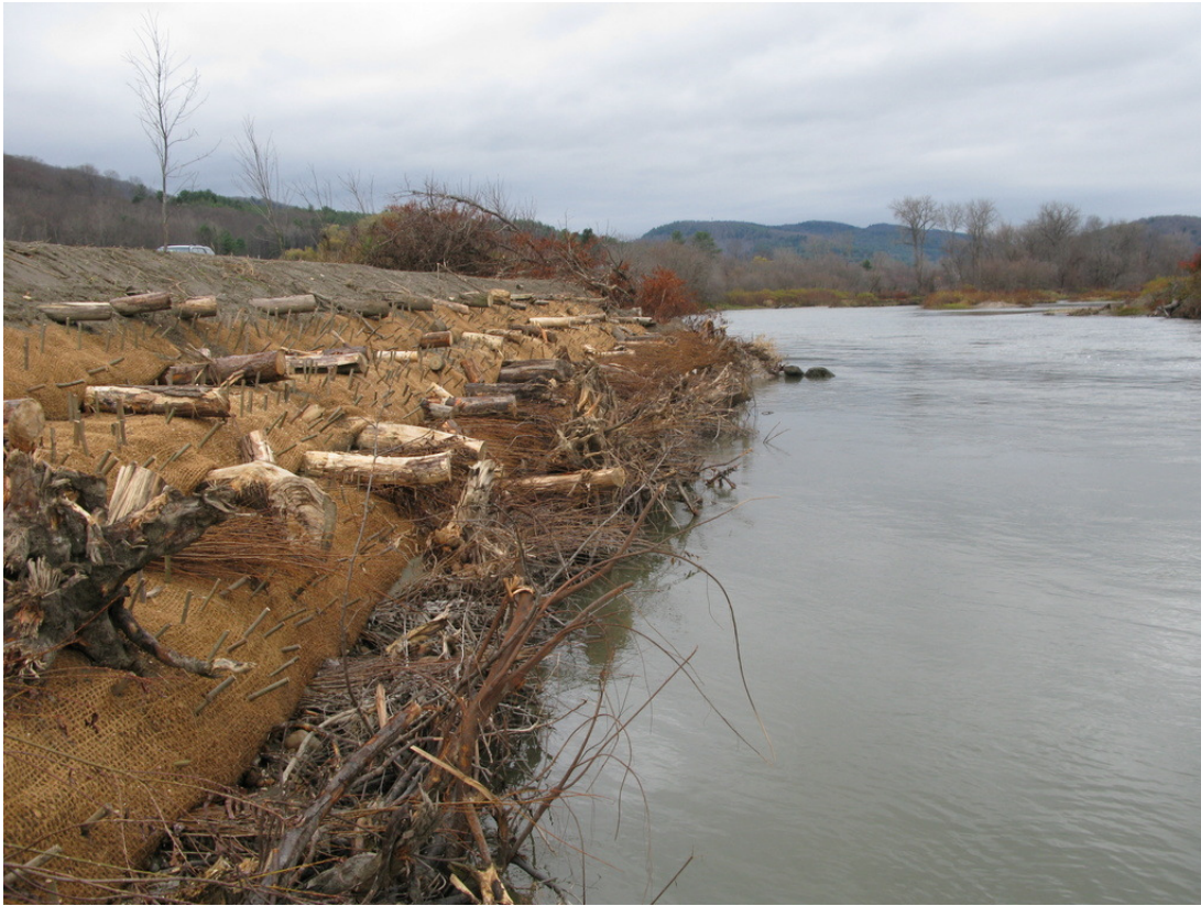
Stage 1 project site during high water flows after Tropical Storm Sandy in November 2012.
