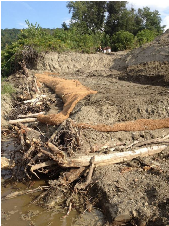
Cross-section view of project site: scour log and root wads covered with a soil lift.
