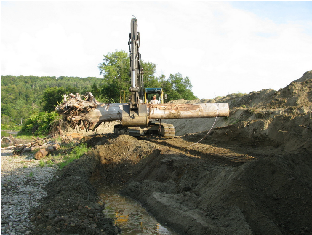
Putting a root wad in place (with deadman anchor cable attached to back end).
