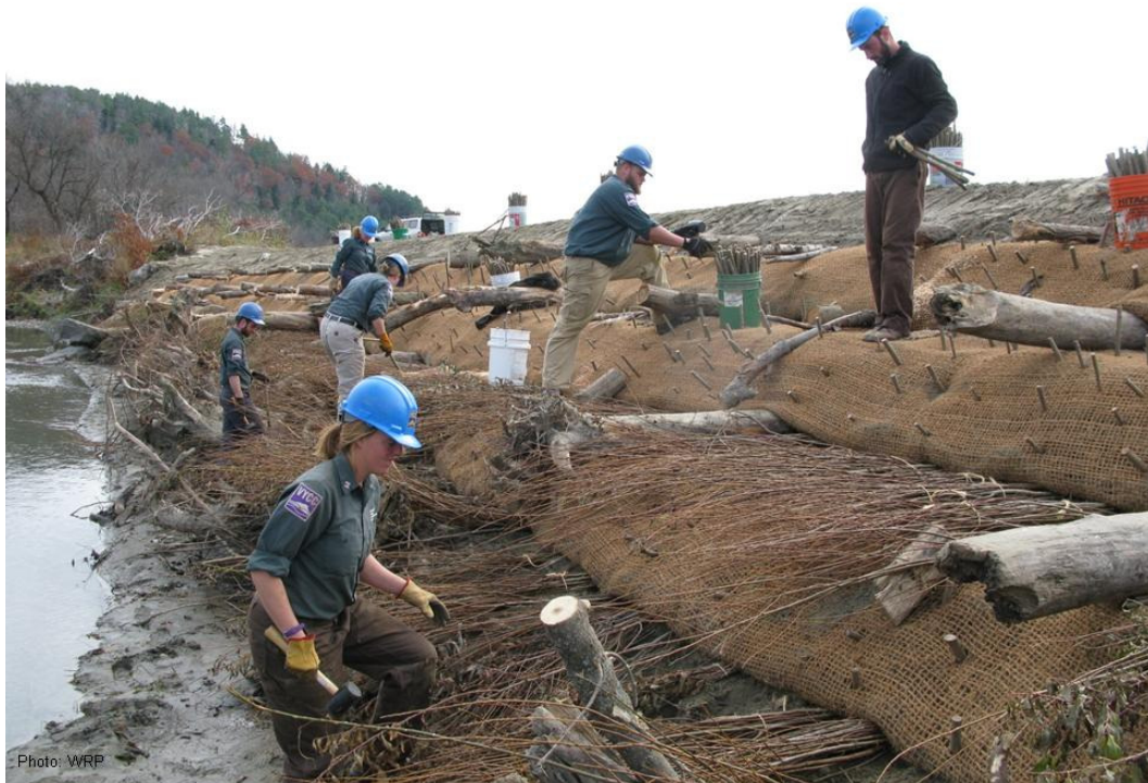
Pounding shub willow stakes to hold the coir fabric in place at the Stage 1 project site.
