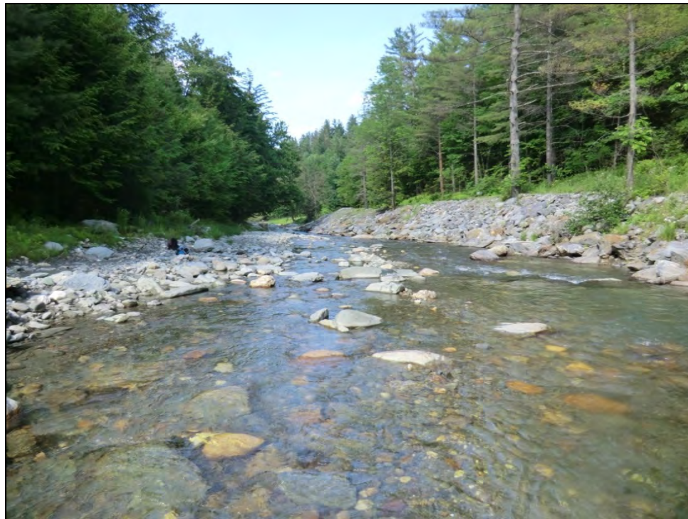
Figure 5.31. Bank armoring along Stony Brook Road is extensive in T5.02.
