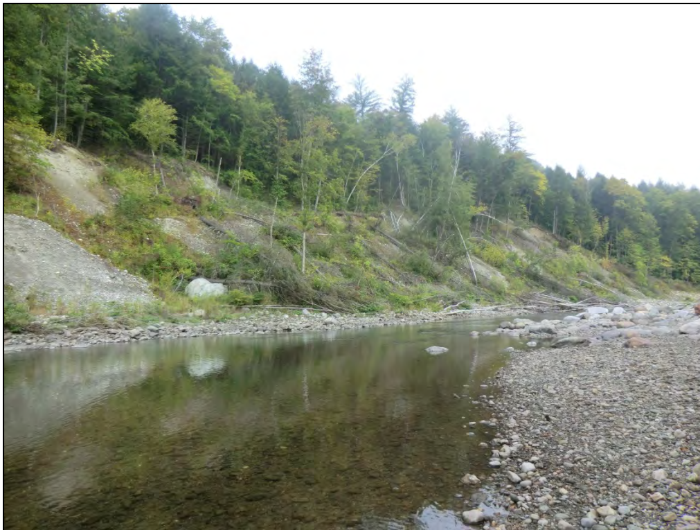
Figure 5.22. Widening has caused mass failures and bank erosion along the White River in R16-A.
