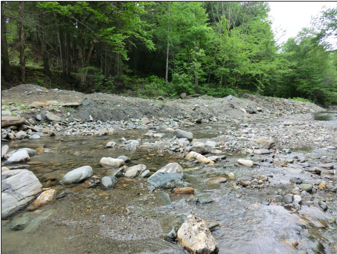
Figure 5.9. Chateauguay Road washed out during TSI in T3.03-B and post-flood work involved windrowing.
