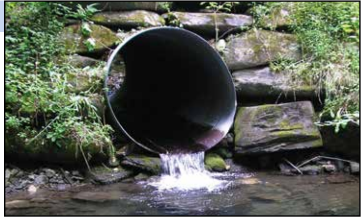
Perched outlet, scour pool and bank erosion.
