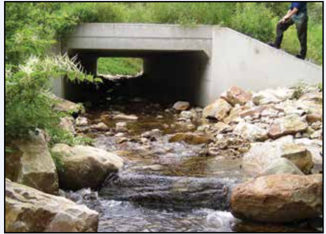
Looking upstream at the new concrete box culvert. Note the rock grade control weir constructed downstream of the project to maintain the streambed elevation at the outlet.
