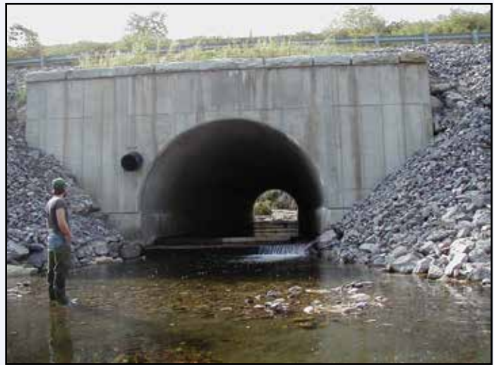
Broad Brook culvert with outlet perch.
