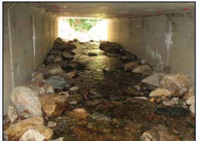
Stream substrate within the culvert was constructed to mimic natural stream conditions and withstand the forces of high flows.
